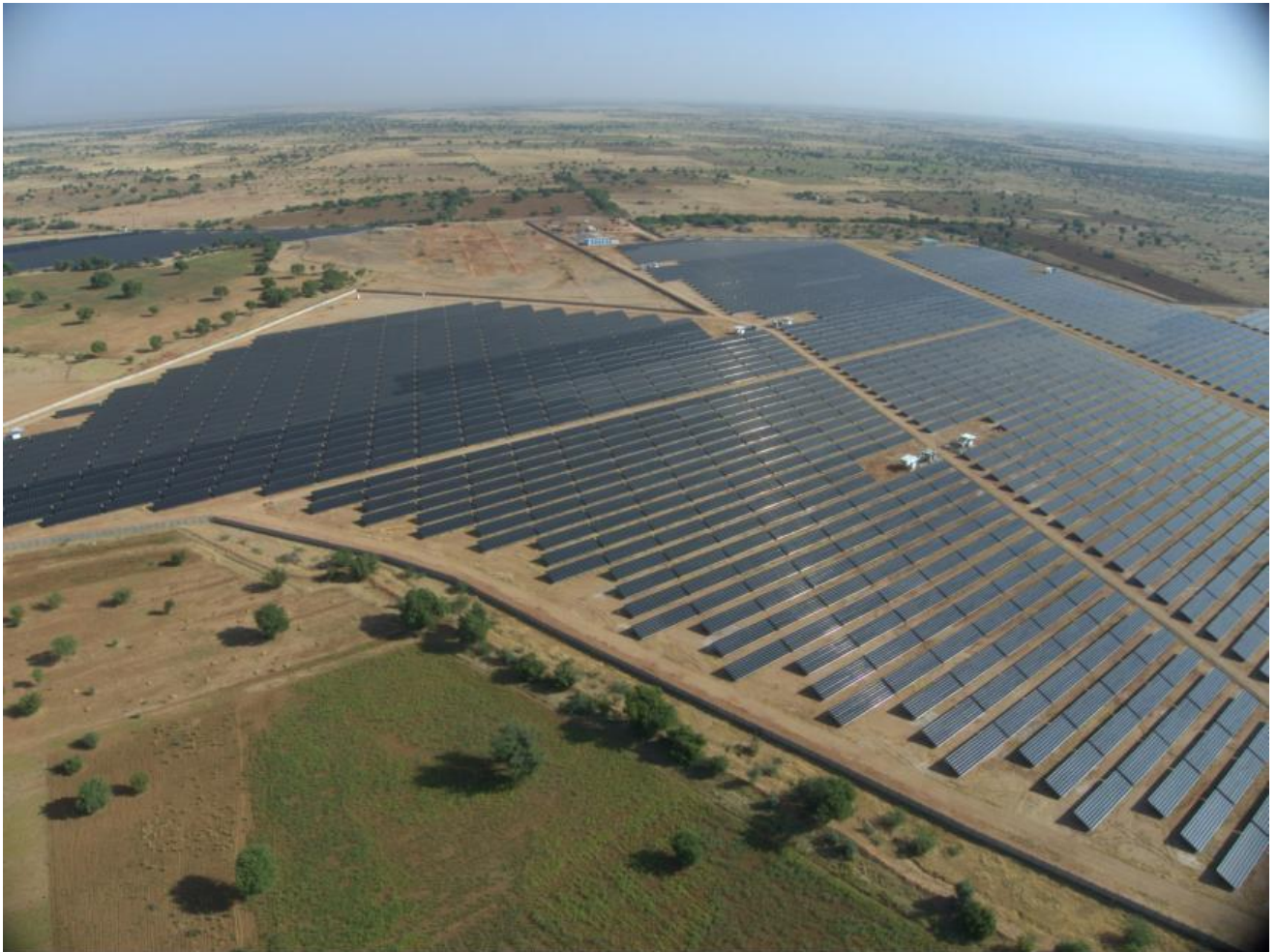
26.44MWp, free-field PV power plant, Jodhpur, Rajasthan
