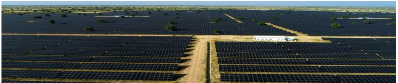
24MWp, free-field PV power plant, Jodhpur, Rajasthan
