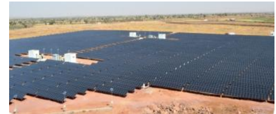
5.2MWp, Jodhpur, Rajasthan, Commissioned in 2011
